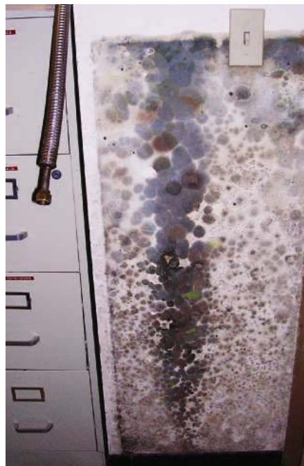
Fungal fright. Mold in a basement chemistry lab at Tulane.
